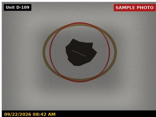
Unstable ceiling surface over shower
