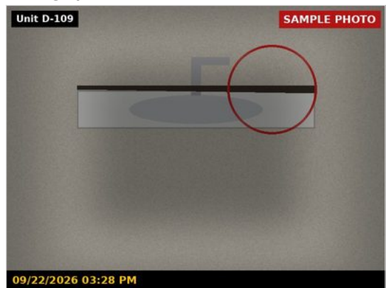
Sink pulling from wall
