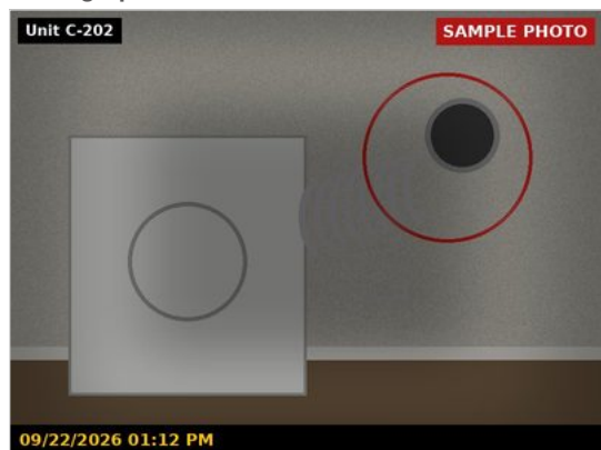
Transition duct detached
