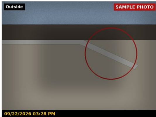
Detached gutter - Bldg D
