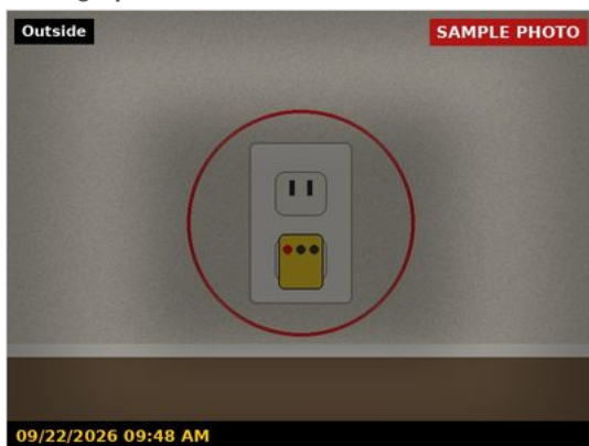
Exterior GFCI fails to trip
