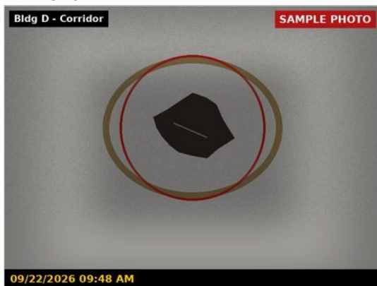
Hole in ceiling
