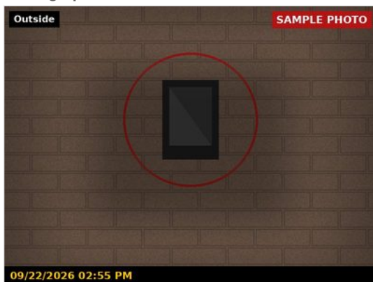
Fixture inoperable - Bldg C entry
