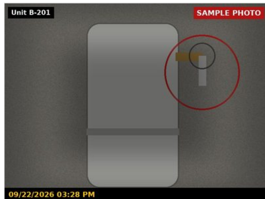
TPR discharge capped
