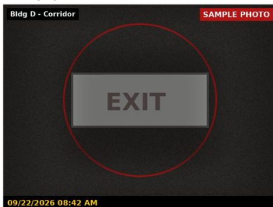
Exit sign not illuminated
