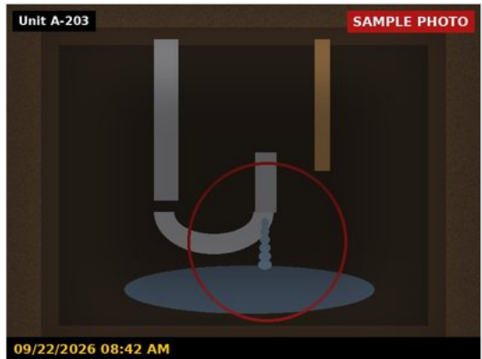
Cabinet floor damage
