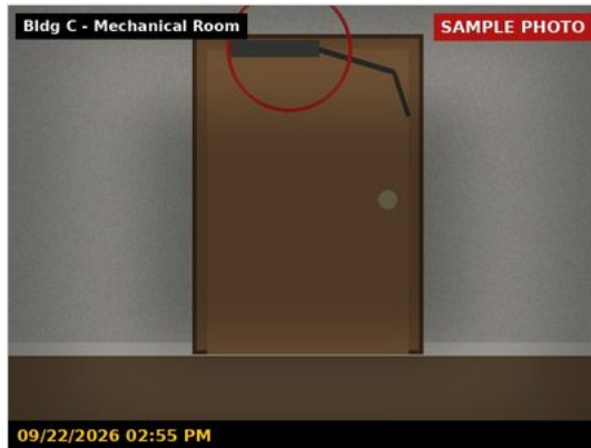
Closer arm disconnected
