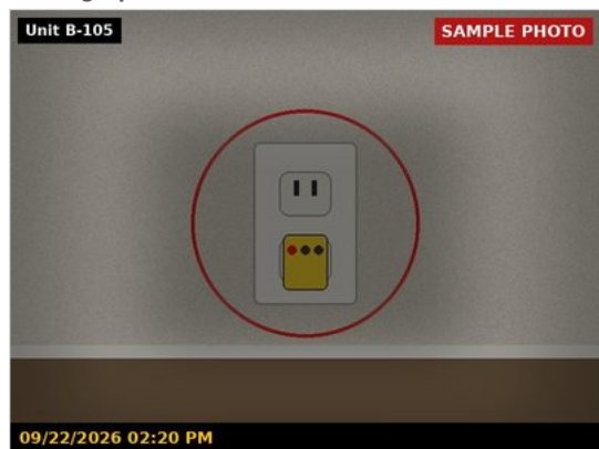
GFCI fails to trip
