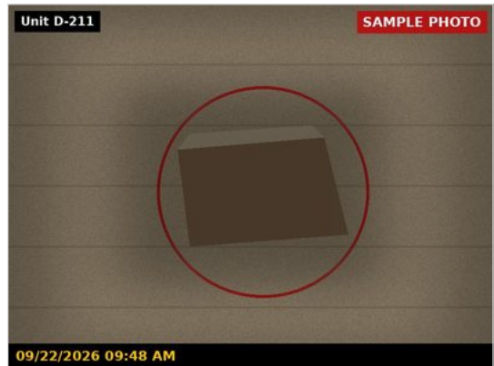
Floor substrate exposed
