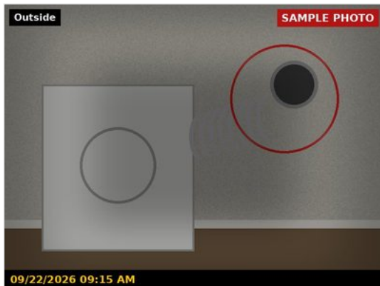
Vent cover missing - Bldg B
