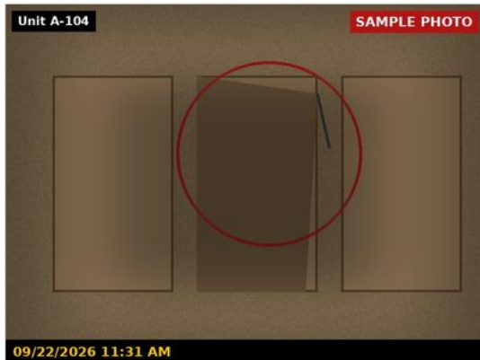
Cabinet door detached
