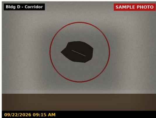
Hole in corridor wall
