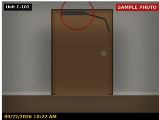
Closet door off track
