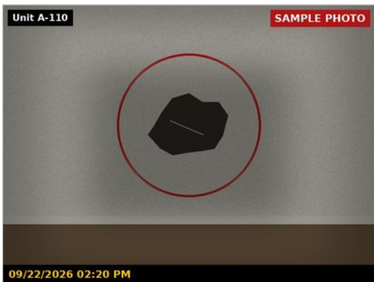
Hole behind entry door
