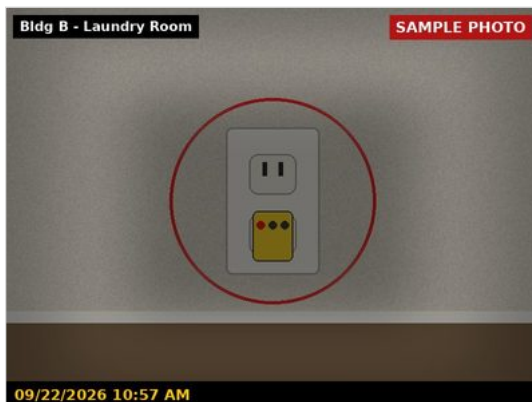
GFCI fails to trip
