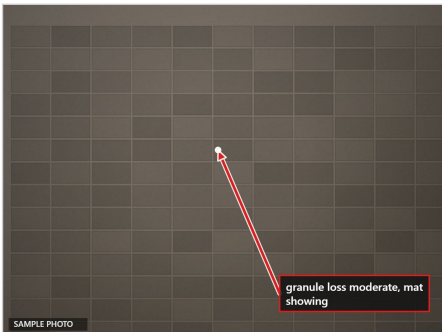
West slope - granule loss moderate, mat showing (2 of 4)
