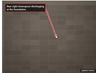
Rear right downspout discharging at the
