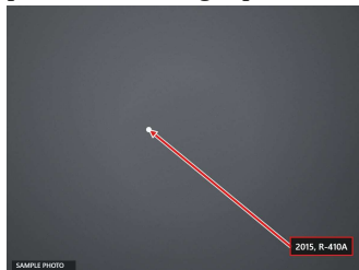
Condenser data plate - 2015, R-410A
