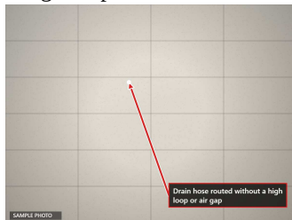
Drain hose routed without a high loop o
