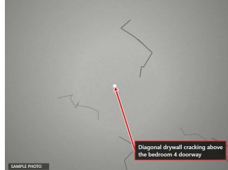
Diagonal drywall cracking above the be
