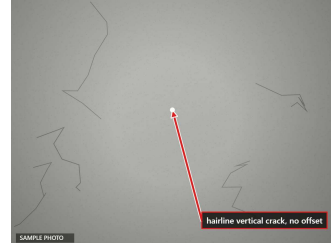
Slab edge, rear right - hairline vertical
